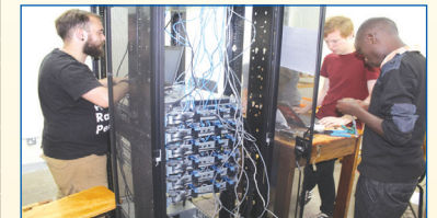
Setting up of the Server Room at Lake Saaka Main Campus.
