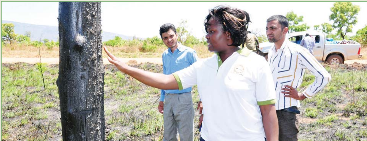
Eng. Deborah Nantume inspecting a burnt electric pole in Karamoja Sub-region.
